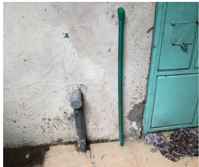
Water pipe to house
